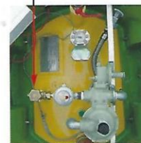
(c) Gas isolation valve
